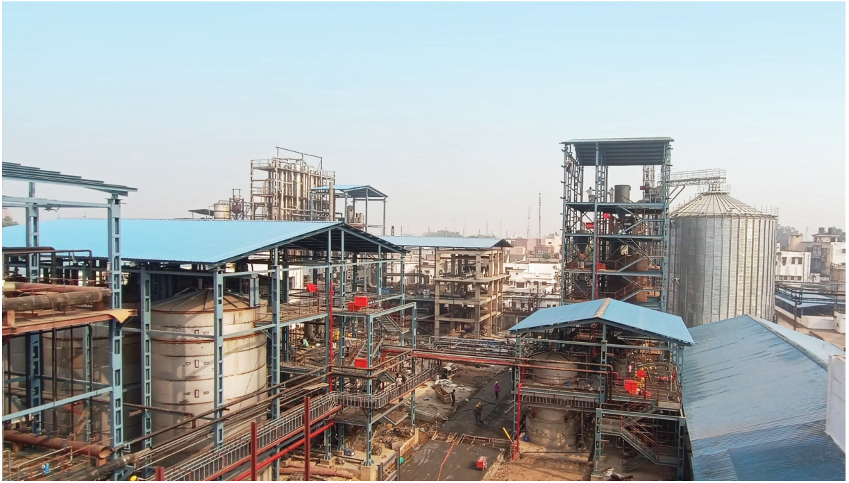
Grain Distillery under construction - Expansion of Modi Distillery. The commercial production will start from January, 2024.
